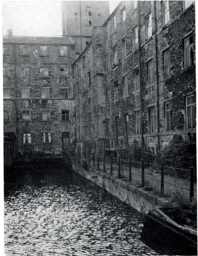
Fig. 8: NORTH AND EAST BLOCKS, LOOKING SOUTH. NOTICE PROJECTING LATRINE TOWER IN NORTH BLOCK (right).
