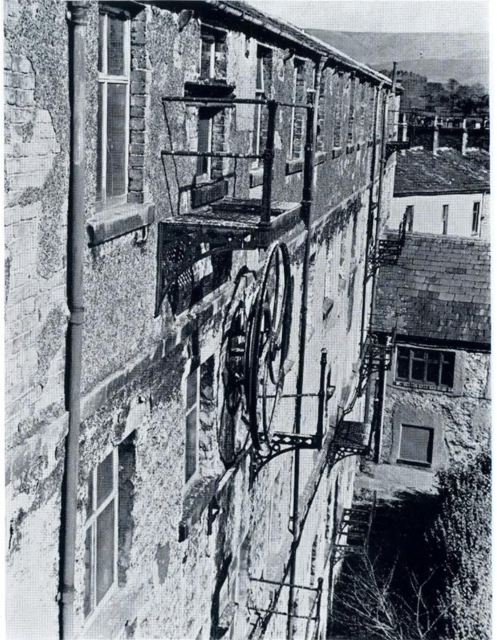
Fig. 10: EAST BLOCK, LOOKING EAST, WITH WHEEL FOR DRIVE FROM MAIN ENGINE HOUSE.
